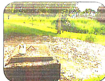
Keep septic tanks sealed.
