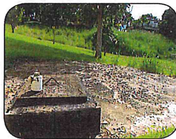
Keep septic tanks sealed.
